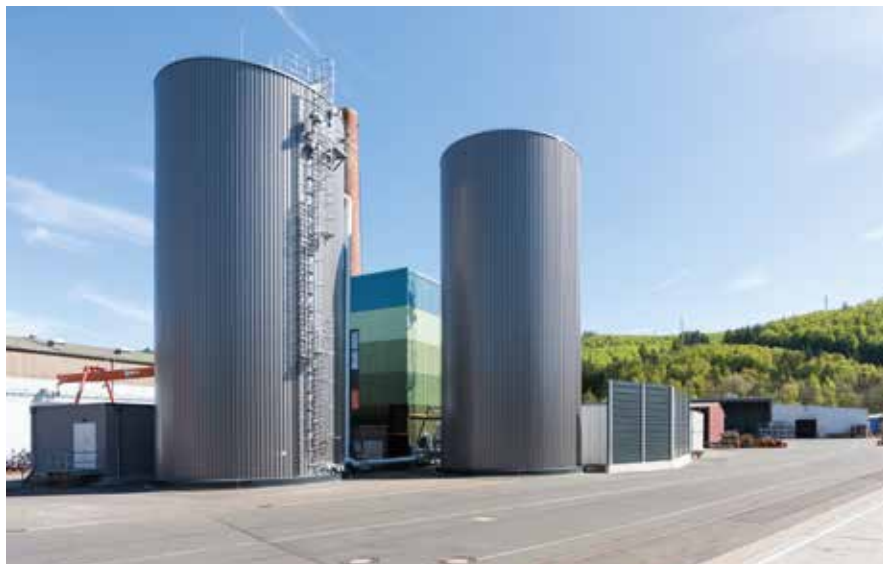
Pufferspeicher (2 x 1.000m 3 ).
